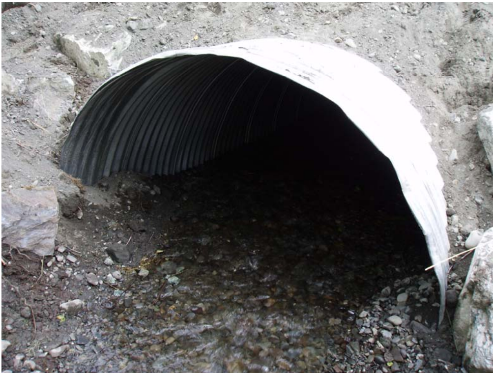
After shot of a newly installed, bedded culvert. A perched and undersized culvert was replaced to improve fish passage on Bean Creek in Cooper Landing using WHIP dollars. (NRCS photo)
