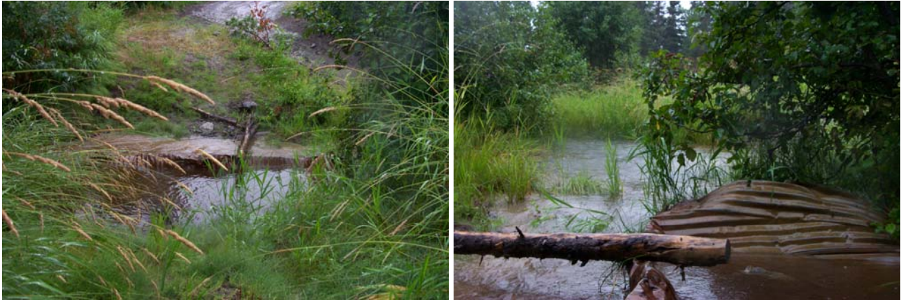
Before shots of Leaf Creek culvert located in the Gray Cliffs subdivision along the North Road Extension. WHIP project will replace the debris and culvert to make more spawning and rearing habitat accessible. (NRCS Photos)
